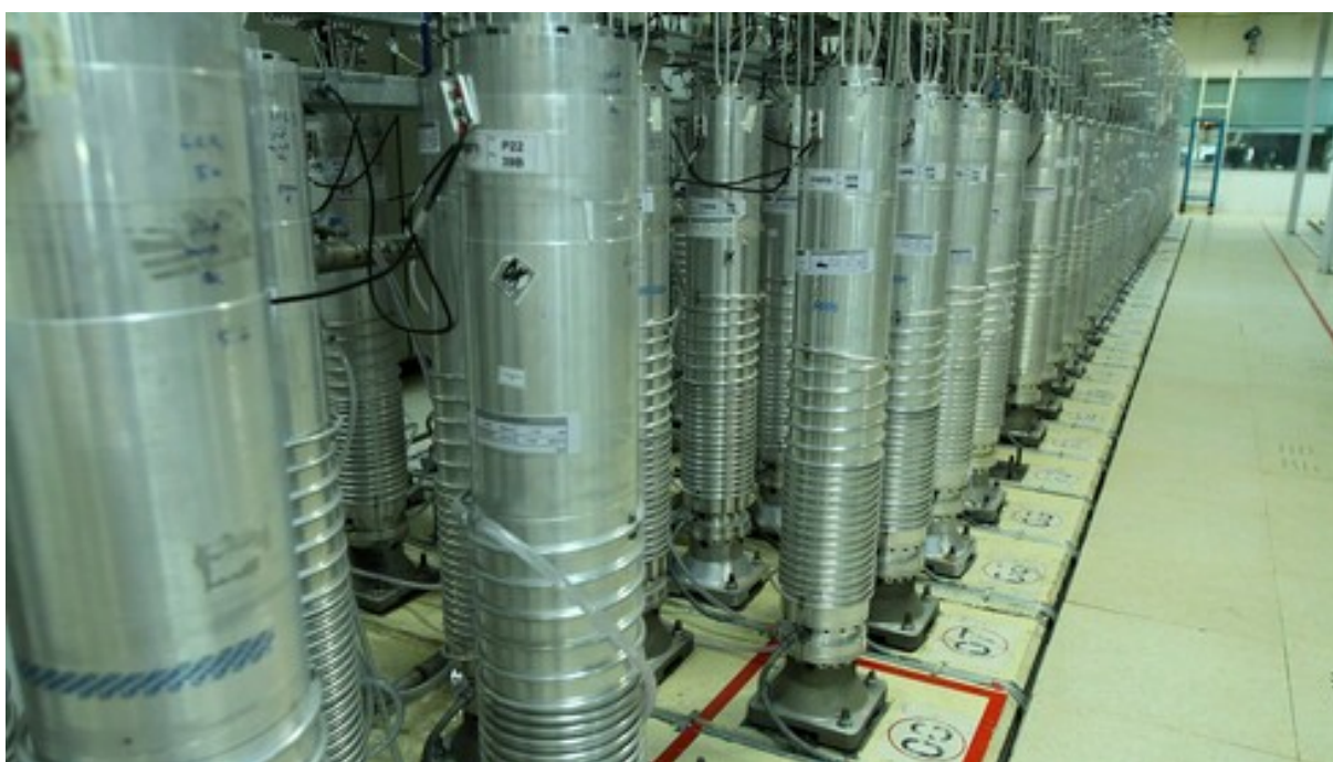
Centrifuge machines in the Natanz uranium enrichment facility in central Iran - (Photo: AP)
