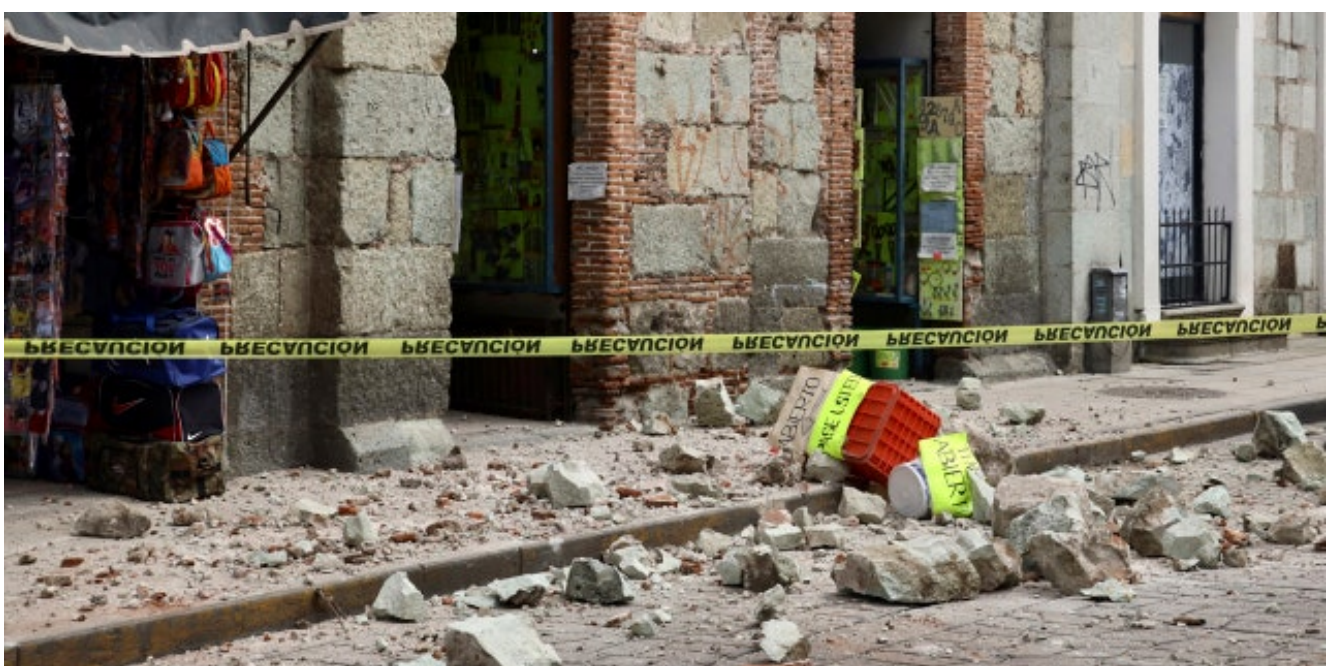
Security tape alert people of a building damaged by an earthquake in Oaxaca,
