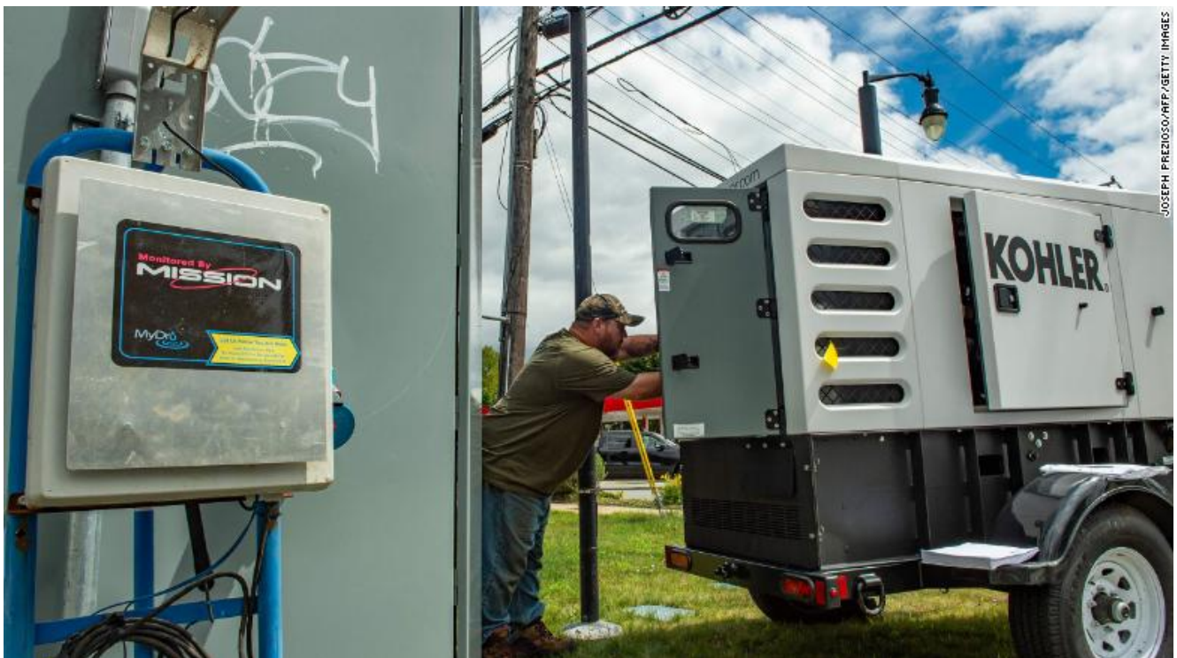
A town employee in Bourne, Massachusetts, connects a generator to a sewage pump in the case of electrical loss as Henri approached Friday.
