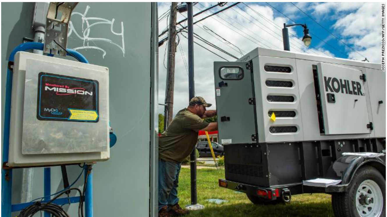
A town employee in Bourne, Massachusetts, connects a generator to a sewage pump in the case of electrical loss as Henri approached Friday.
