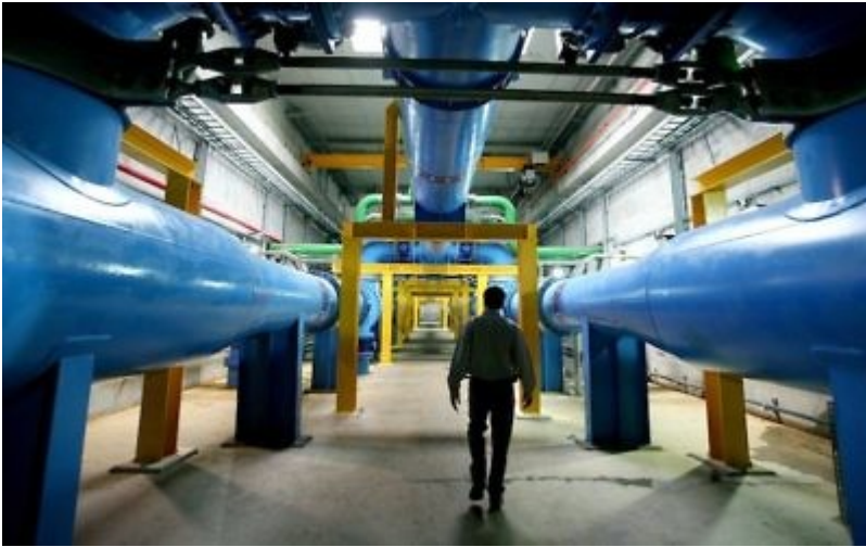
View of the Eshkol Water Filtration Plant in Northern Israel (Moshe Shai/FLASH90)
