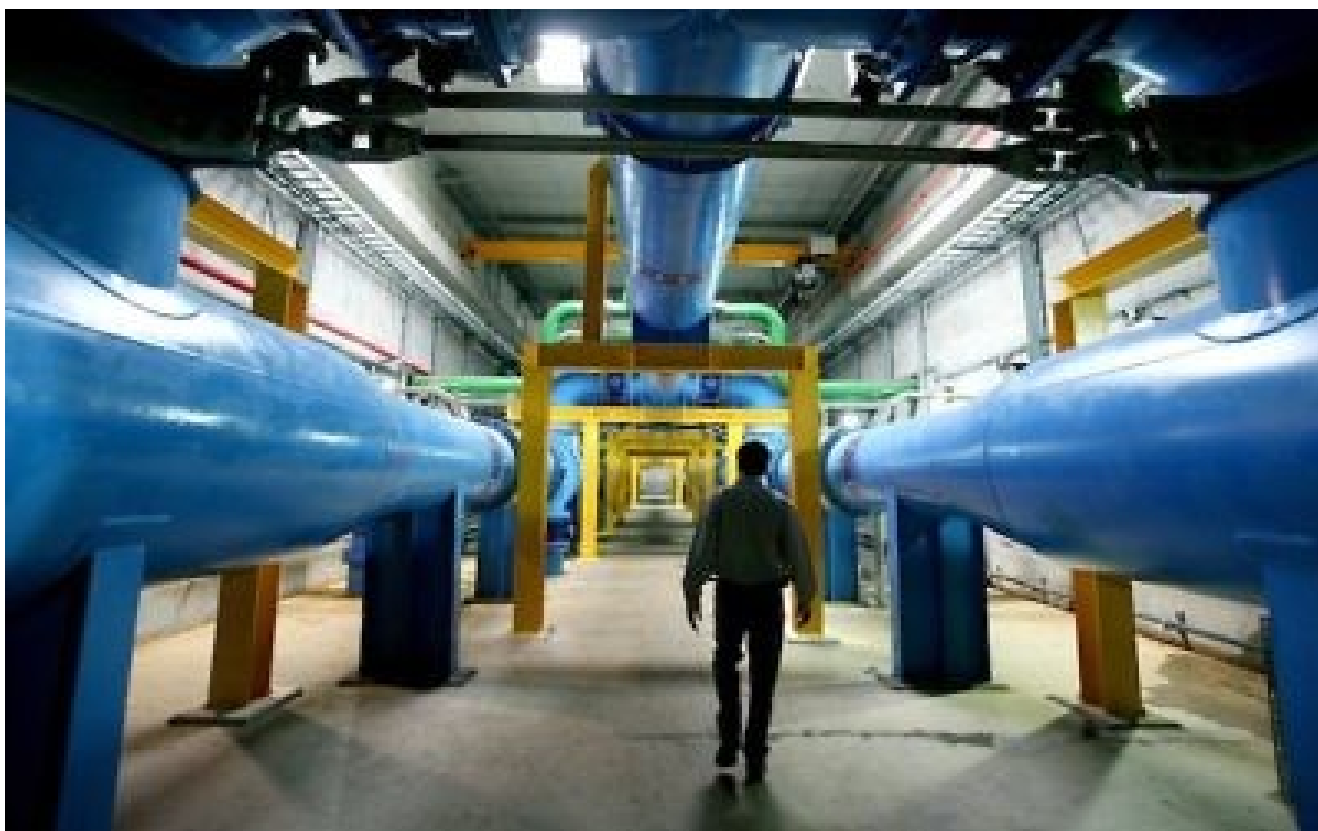
View of the Eshkol Water Filtration Plant in Northern Israel (Moshe Shai/FLASH90)
